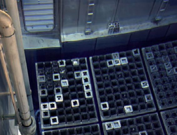
(From left to right) Maintenance work performed on a Diesel engine at an EDF plant / Ten-year inspection of the spent fuel cooling pool at Cattenom unit-3 NPP.
