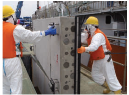
Mounting of the new containment on a damaged reactor at the Fukushima Daiichi power plant.
