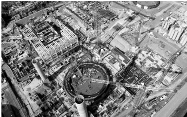
Work in progress at Flamanville (France) where the first EPR-type reactor unit in France is under construction.
