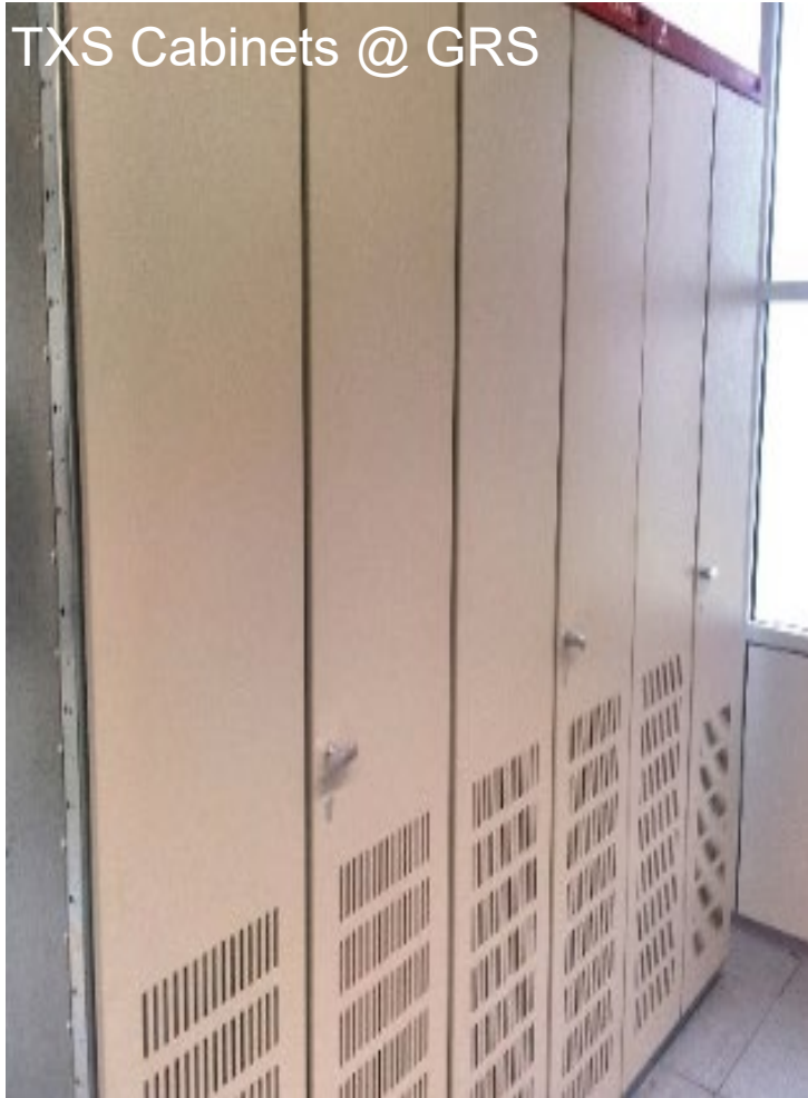
TXS Cabinet - Inside View
