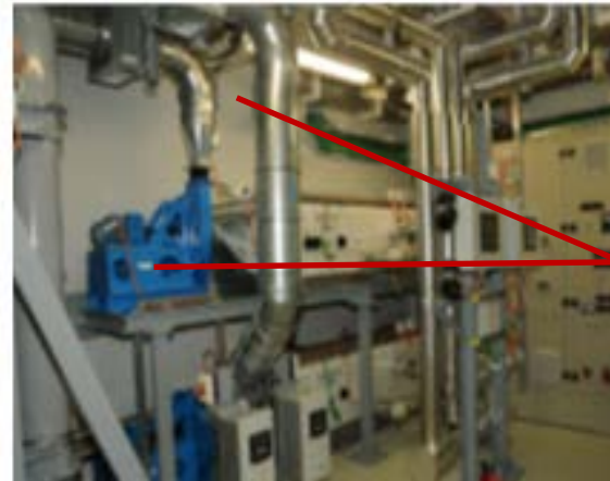
Air conditioning equipment of emergency control room
