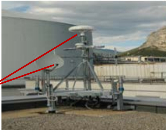
Communication devices (roof of PCS3)
