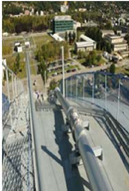
CDS circuit on RB roof
